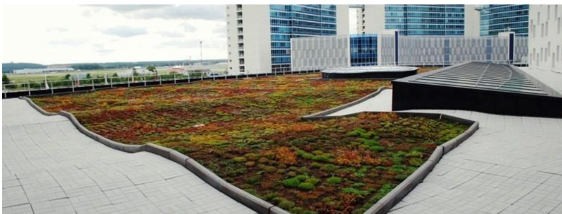
Figure 4.3 Green roof of the multifunctional complex Airport City
