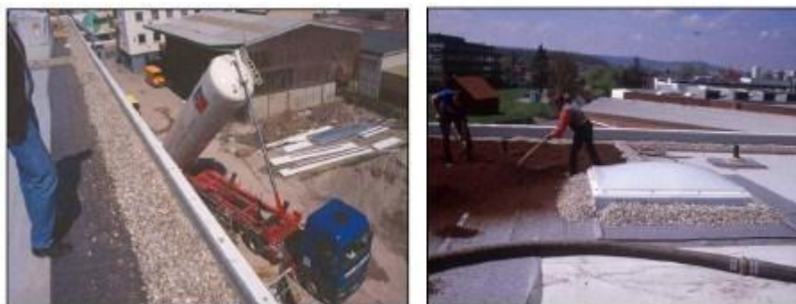
Figure 3.8 Pneumatic conveying of soil on the roof in Germany. On the left - a truck used for transporting the soil to the right - the pump hose is used to supply ground to the roof, and the workers, spread it with a rake ( http://iconroofing.ca/our-services/roofing-repairs/ )
