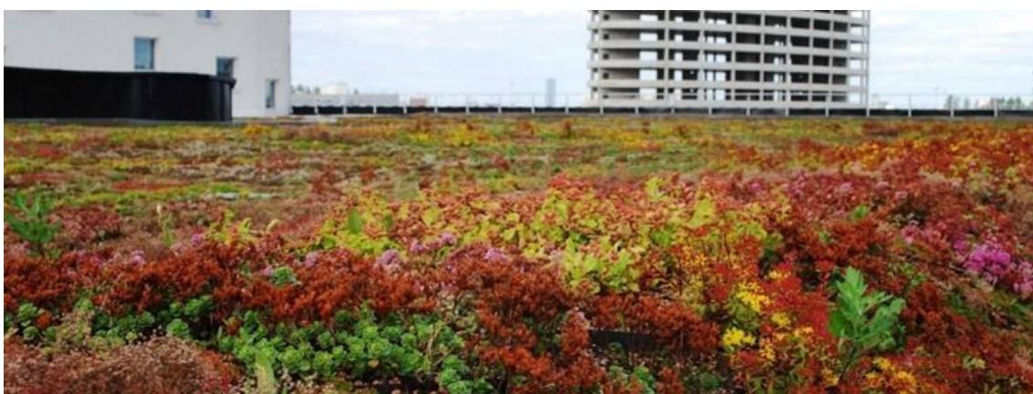
Figure 4.4 Green roof of the multifunctional complex Airport City
