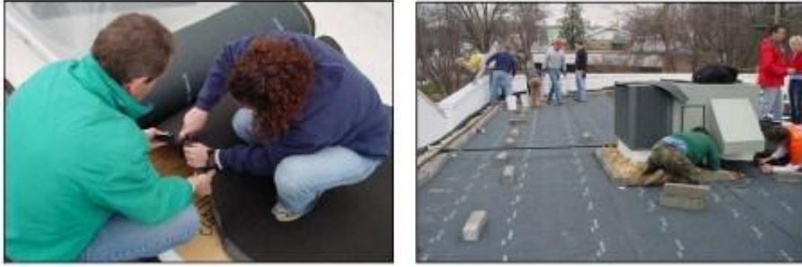
Figure 3.7 Left - cutting protective layers for placing on the roof. Right - laying protective layer before placing on the roof of the soil
