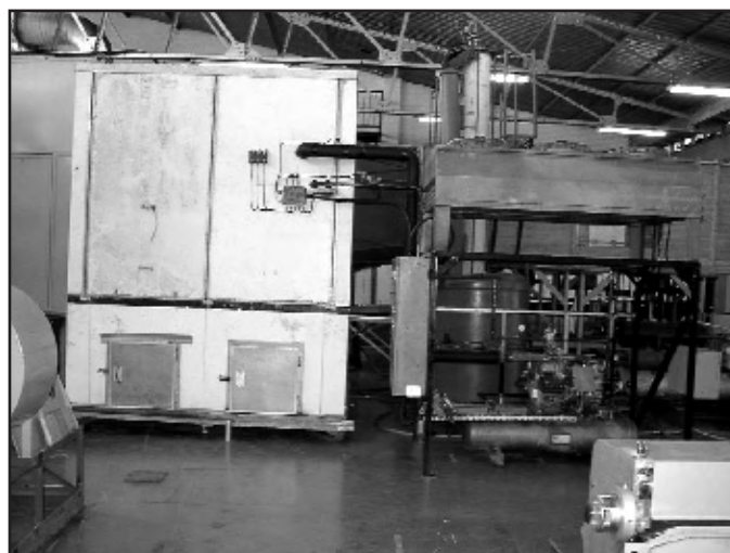
Figure 5: Ice plant at Wits University
