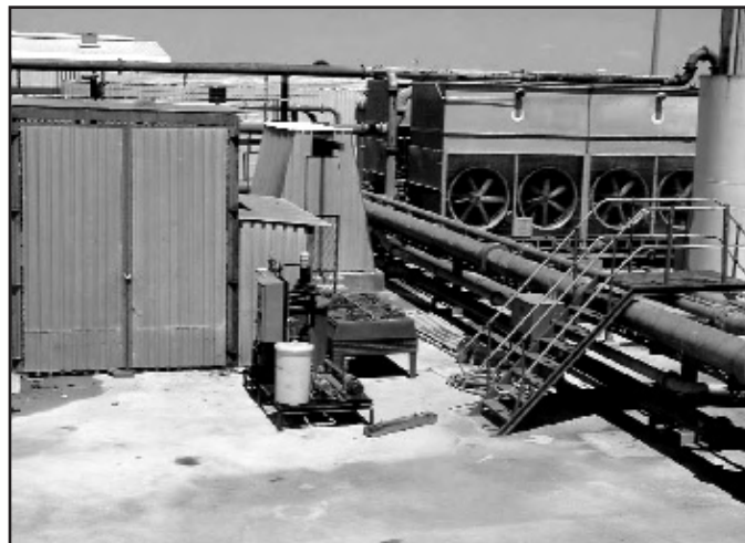
Figure 4: Pilot plant at Driefontein Mine
