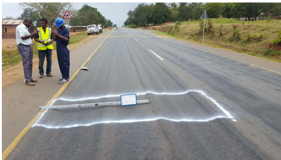
Figure 1: Rutting on the departure from a speed hump.
