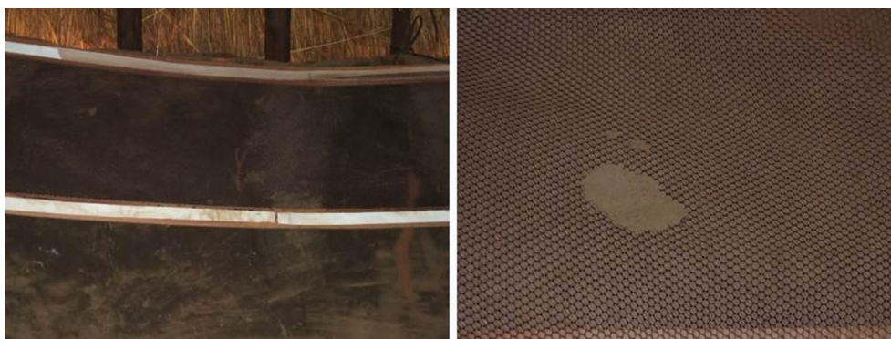
Fig. 3 Water and rodent damage observed on a purple lining installed in a hut during the month four interview. The wall is damp/wet in the darker sections (left). Water damage in the form of brown watermarks can be seen on the Velcro®. A close-up of the rodent damage noted on the lining (right)
