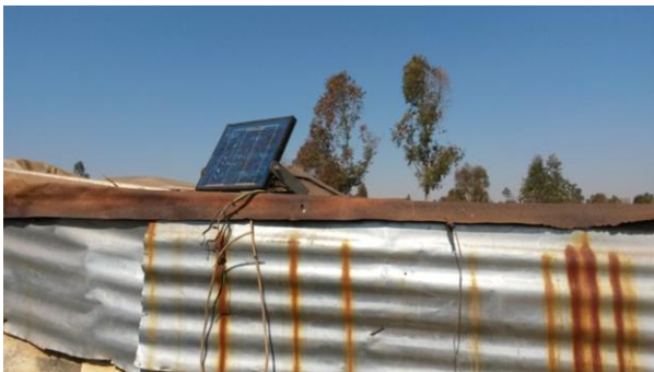
Figure 5. Solar Panel used for a source of power supply (Coetsee.et.al., 2014).[1]
