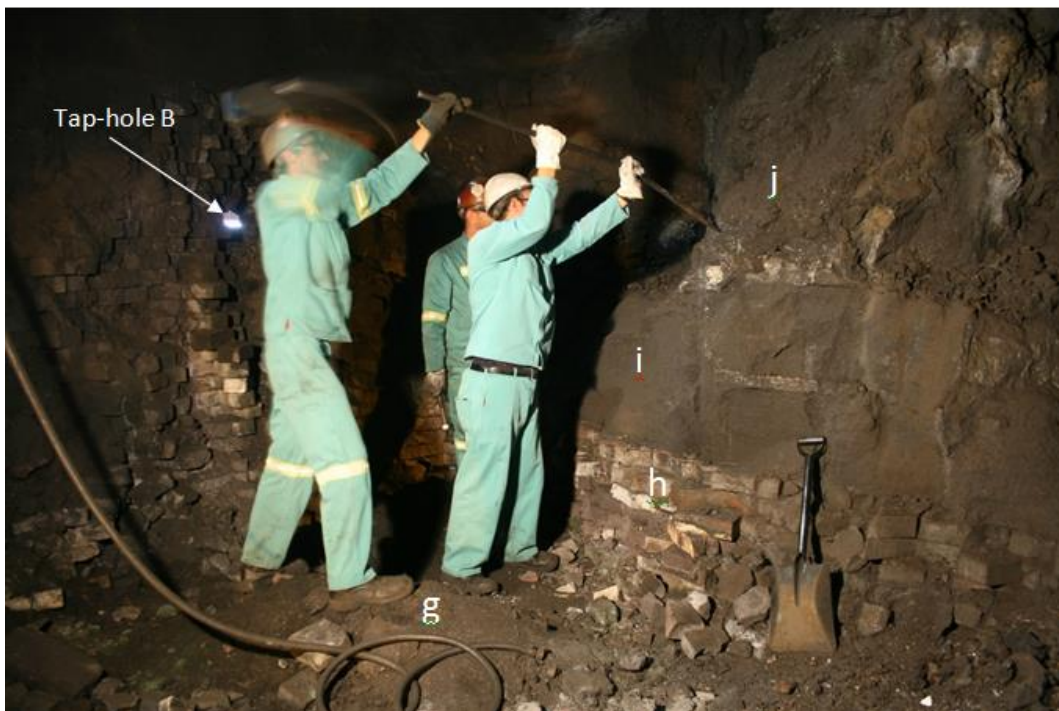
Figure 110: Tap-hole B put into perspective. The operating personnel are standing on (g) the steel shell / fireclay castable of the furnace hearth sampling the metal layer at the interface between the (i) high grade carbon ramming and (j) burden. Also note the (h) five layers of super duty fireclay bricks in the hearth.
