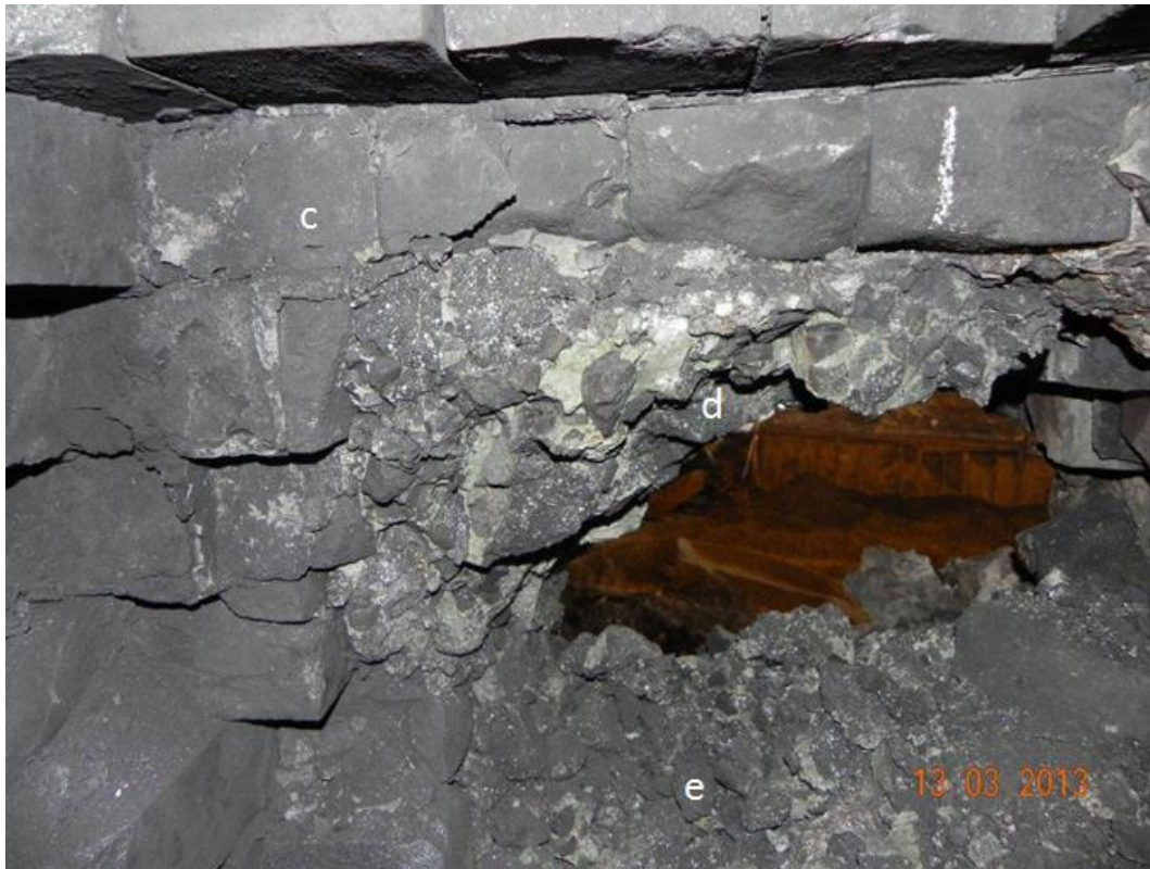
Figure 109: Tap-hole B with (c) SiC bricks, (d) slag with burden and / or coke bed material and (e) mixed material containing metal.
