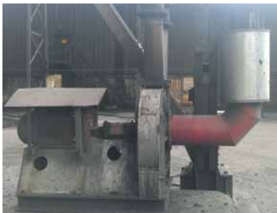
Figure 5. Silencer fitted on a fan exhaust resulted in 11 dB(A) reduction in noise level
