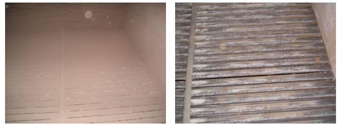
b) Fouled and cleaned tube bank
