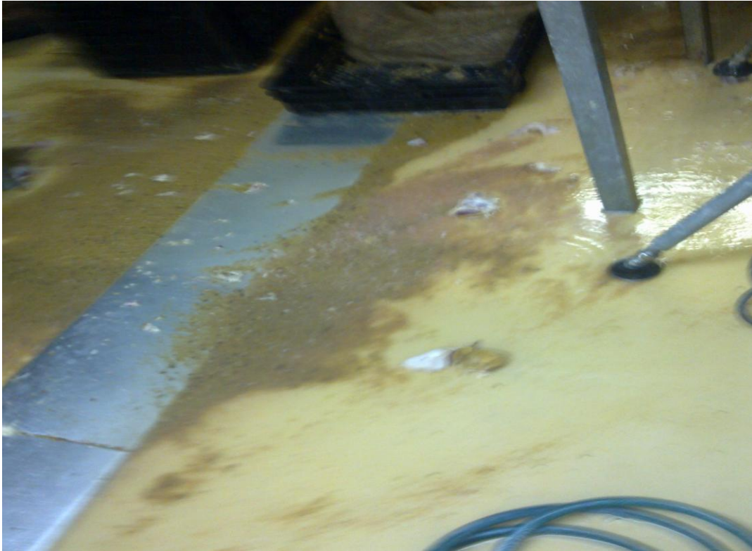
Plate 4.18: Deficient drainage of waste water and feces
