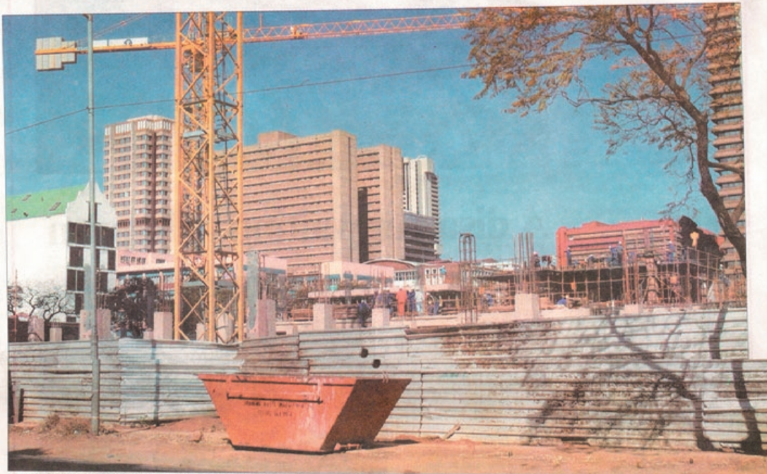
□ The Department of Public Works and the Tshwane Metro Council are working together to ensure the country has a capital city its people can be proud of. Construction has started on the new National Library in Andries Street.
