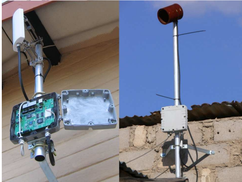
Figure 6.2: Outdoor mesh node with repackaged Linksys WRT54G electronics in a waterproof aluminium case. The picture on the left shows an installation at node D is using a commercial 8dBi flat panel, the picture on the right shows an installation at node H which is using a home made Cantenna.
