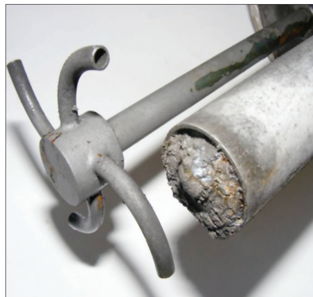
Figure 4—Blocked feed tube
