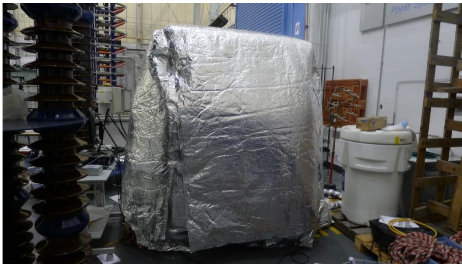
Figure 4-22 The transformer after being wrapped with insulating jacket
