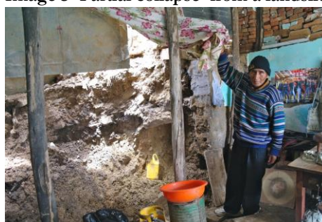
Image 3 'Partial collapse' from a landslide
