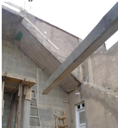
Image 20 Section of the retaining wall that the Municipal House constructed in Vinateros following the landslide in 2006
