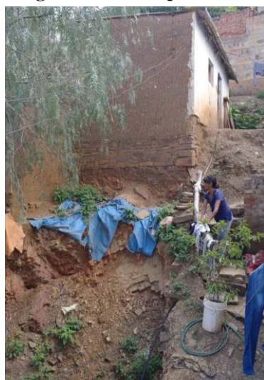
Image 2 'Total Collapse' from a landslide
