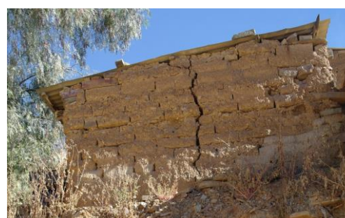
Image 5 Cracked walls due to water damage
