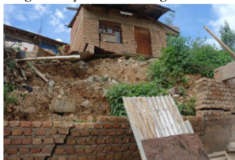
Image 4 'Very serious' damage from a landslide
