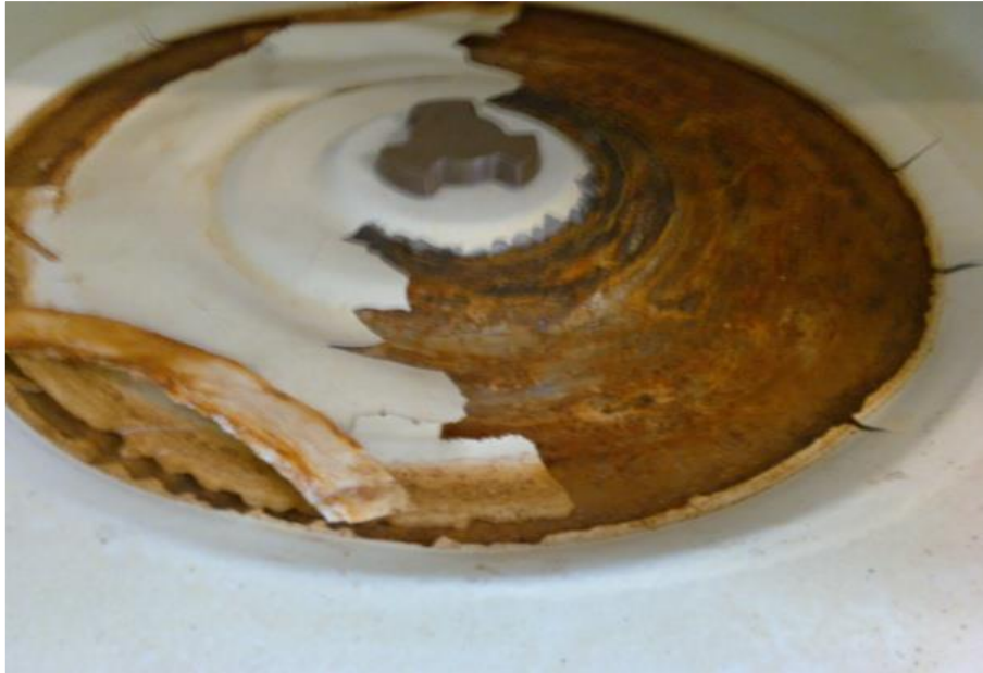
(a) Cracked paint
