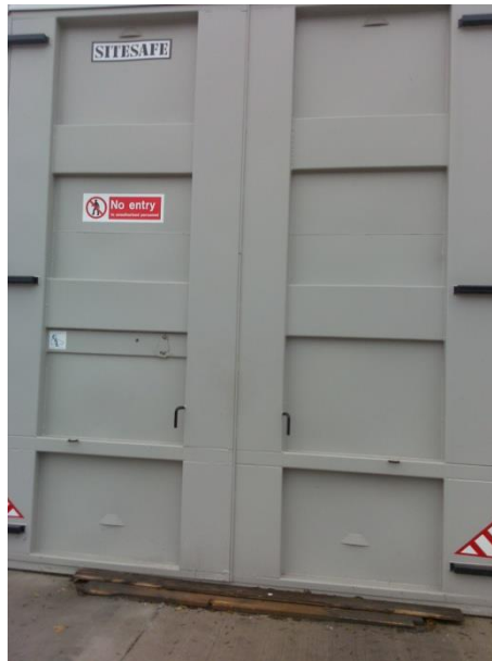
Figure 4.5: The container allocated by VLGM to conduct a fault diagnostic study by researchers from the University of Manchester.
