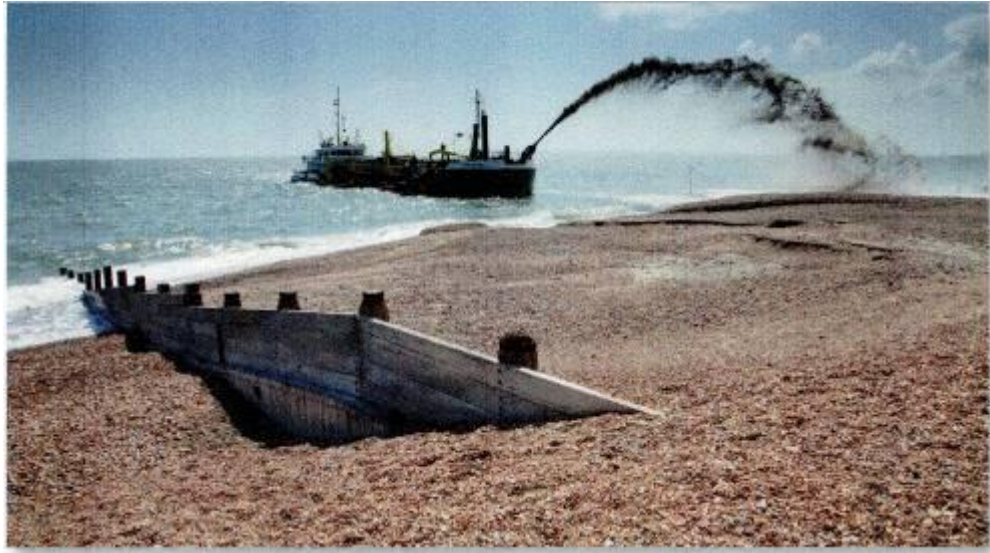
Fig. 5.4: Beach nourishment on Hayling Island, Hampshire. (From James et al. 2011, 13).
