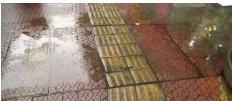
Figure 8.66. The inappropriate pavement material in Haier Xiang
