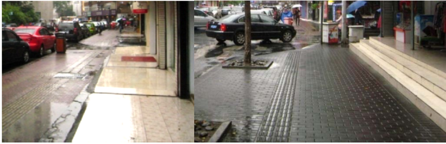
Figure 8.67. Different conditions of the footways in the western (left) and eastern part (right) of Haier Xiang
