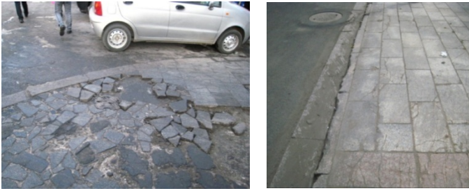
Figure 8.13. Pavements damaged by heavy vehicles in Dazhi Street (left) and in Chengnan Road (right)
