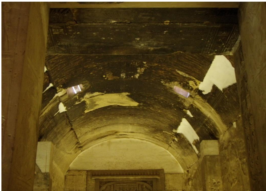
Figure 1.21: Roof of Seti I's temple at Abydos showing soot deposits on the vaulted roof (Author's own photo). The lighter areas are modern restorations of the roof.
