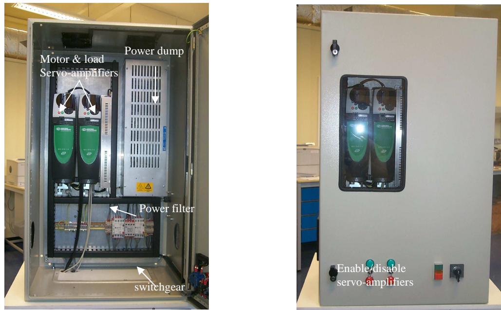
Fig. 3.12 The Unidrive motor drive system [1].
