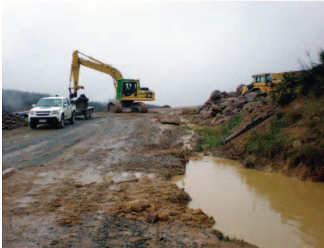
Sediment in a silt trap at an earthworks operation in Canterbury
