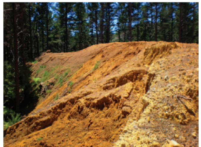
Erosion of exposed fill slope on a landing in the Waikato
