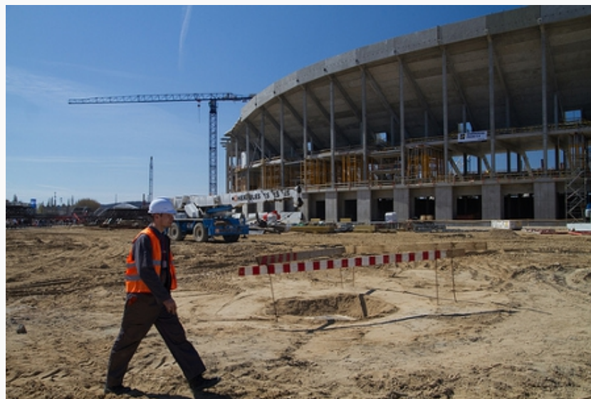
PGE Arena Gdańsk under construction in 2010 Credit: Adam Kuśmierz (Creative Commons BY ND)
