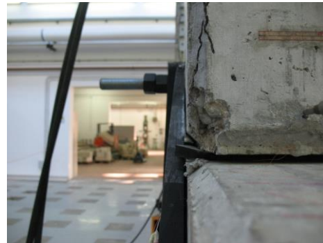
Fig. 18 Neoprene pad deformation (test 2)
