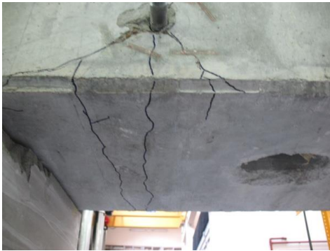
Fig. 13 Cracking pattern on the West side-bottom surface of the beam (test 1)
