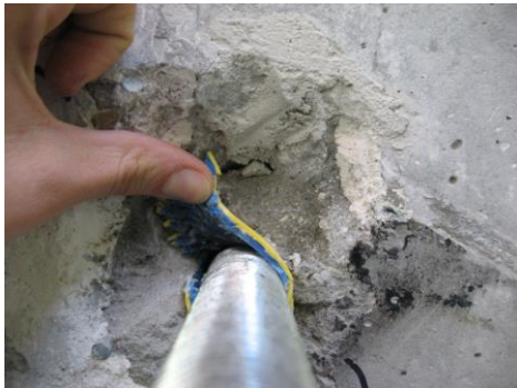
Fig. 17 Rubber hose damage (test 2)
