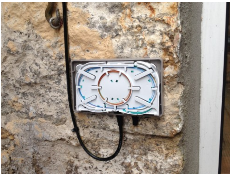
Figure 3.14: A Typical FTTP Installation Showing Coiled Fibre-Optic Cable Ready for Termination in a Customer Premises
