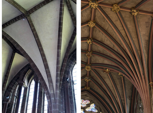
Figure 1 Vaults from the Chester Cathedral Chapter House (left) and Exeter Cathedral Lady Chapel (right) for the large scale investigation.
