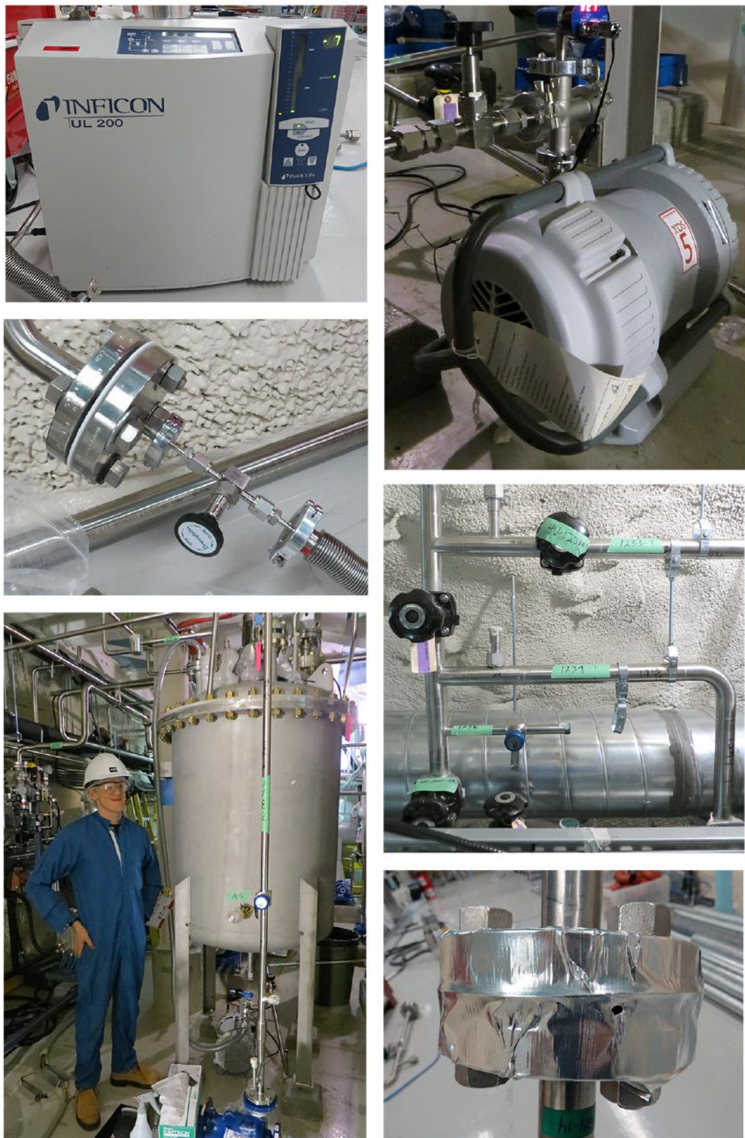
FIGURE 3.21: Top-left: helium leak detector and vacuum pump. Top-right: scroll vacuum pump. Middle-left: needle valve. Middle-right: pipelines and hand-valves. Bottom-left: author beside vessel. Bottom-right: joint sealed with aluminium tape, a hole is pierced in order to inject helium.
