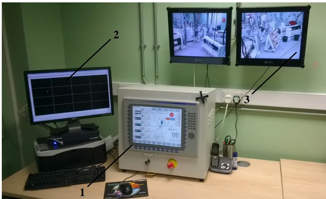
Figure 4.9: The control room featuring a HMI at “1,” a monitoring PC at “2,” and video feeds of mixer facility at “3.”
