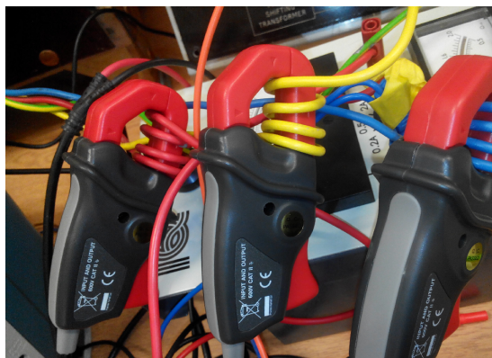
(b) Three current clamps installed
