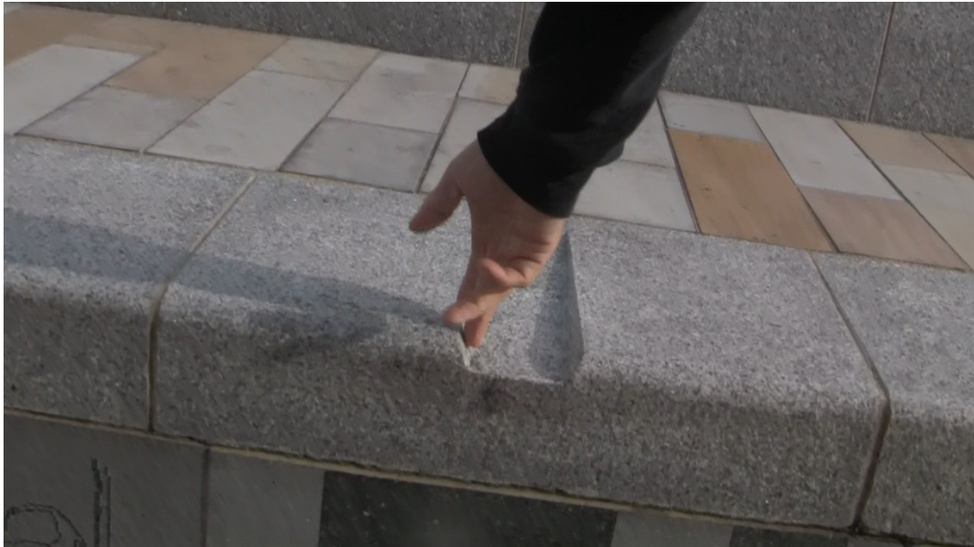
Figure 66 – Indents within stonework demonstrate the existence of strategies embedded within architecture to prevent activities such as skateboarding (17, Q on map).
