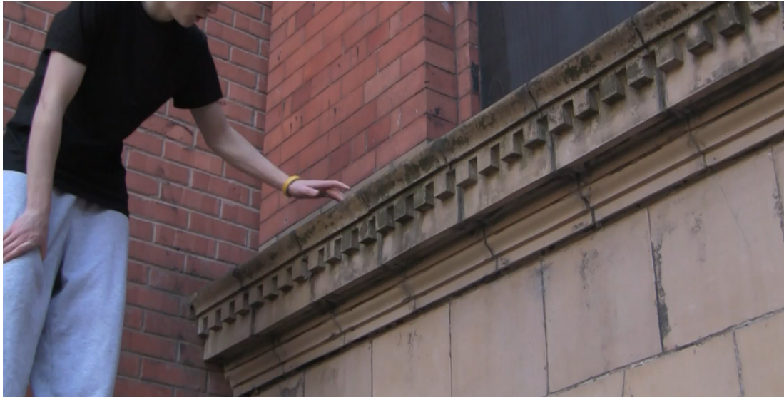
Figure 92 – Vandal grease that is used to prevent access to specific surfaces, presenting a potential danger to traceurs (14, J on map).
