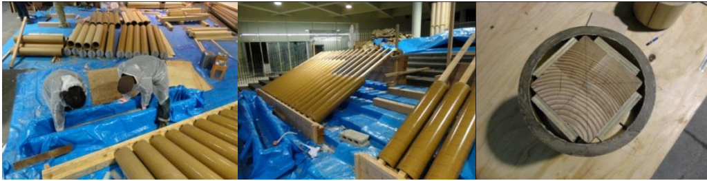
FIGURE 2.41. - 2.43. Two volunteers soaking a paper tube in the fire proof paint; Paper tubes after treated with fire proof paint; Timber inside a paper tube to support the tube structure 129
