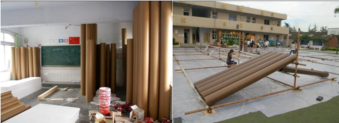
FIGURE 4. 33. - FIGURE 4. 34. Paper tubes being stored inside a classroom in the concrete building; Paper tubes being treated by waterproof paint 37
