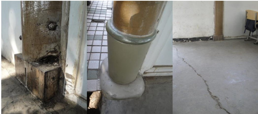
FIGURE 4. 35. - FIGURE 4. 37 The end of a paper tube was damaged by the rain; The metal replacement; A crack appeared on the floor in one of the classrooms
