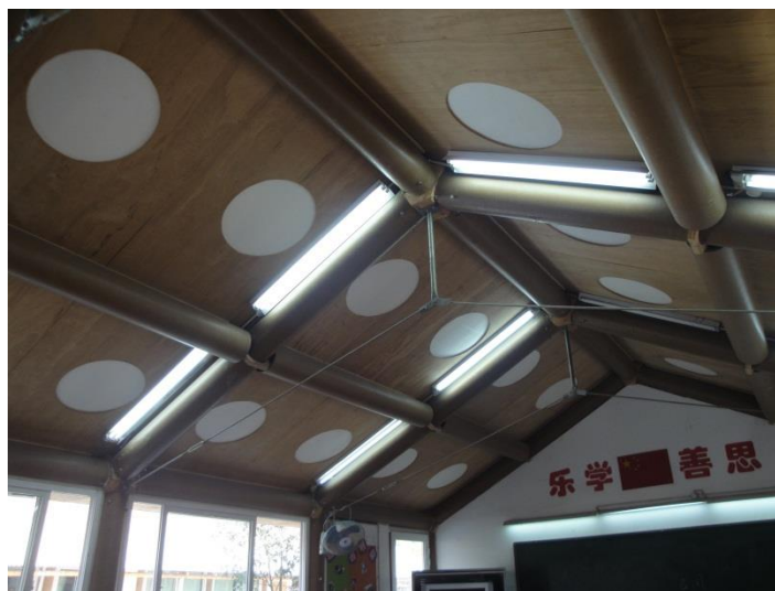
FIGURE 4. 21. The fluorescent lights on the ceiling in one classroom
