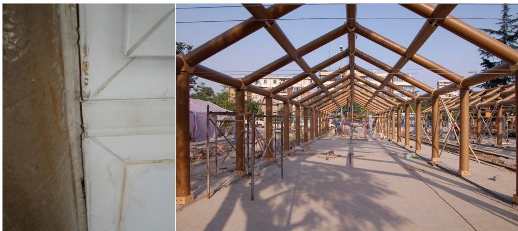
FIGURE 4. 41. - FIGURE 4. 42. The crack shows that the PVC door and the paper tubes are detached; The frame structure of the building 43
