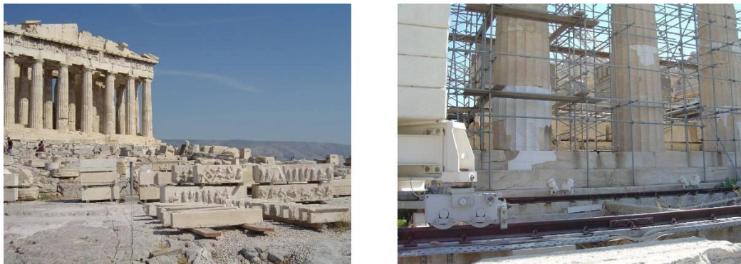
Figure 2.6: The Parthenon in Athens. From a distance, the visual difference between original and new material is minimal (left). On closer inspection, differentiation between original and new materials is revealed (right). Image credits: André Brown.
