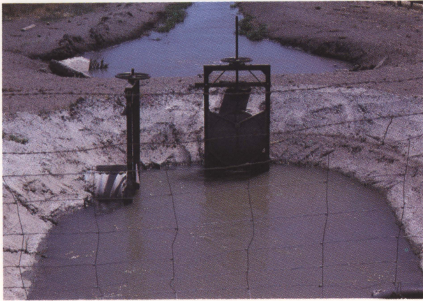
It may be necessary to install concrete aprons around headgates and tubes to prevent muskrats from burrowing next to them.
