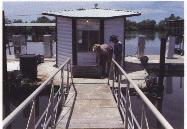
Damage to the flotation supports cause the houses and docks to tilt or sink; repairs are quite expensive.
