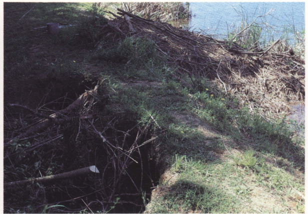
These beaver tunnels are in a man-made dam built to impound water. Such tunnels commonly cause failure of dams, loss of water and costly repairs.
