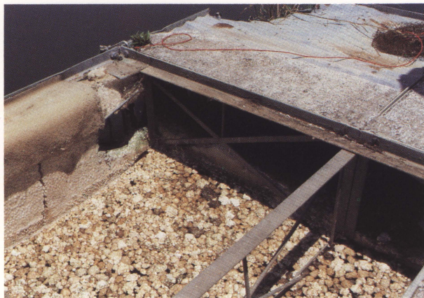
This type of beaver damage to styrofoam and wood supports under boat houses and docks is a frequent reason for complaints from marinas.
