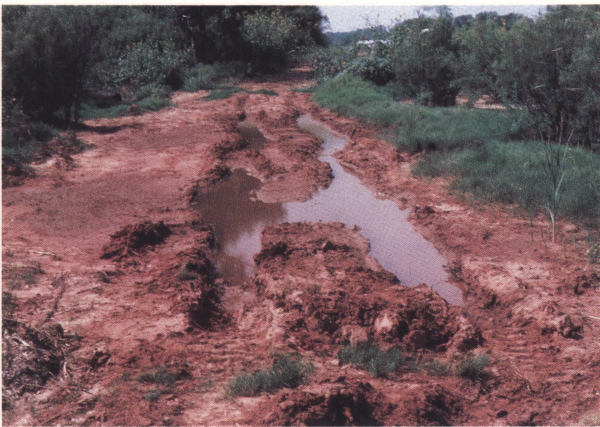
Roadway flooding often occurs near beaver ponds.
