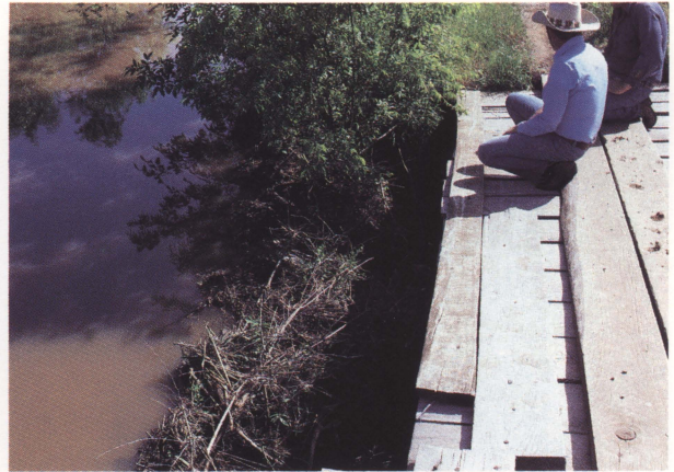
A bridge opening, dammed by beaver, caused flooding of the roadway.
