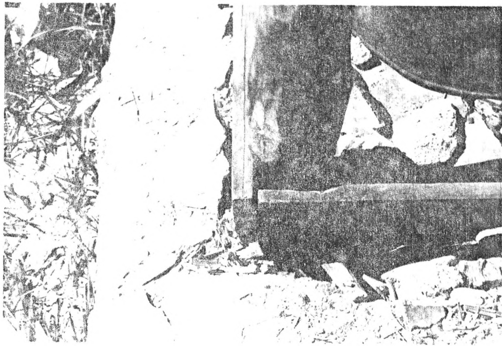
Figure 11 - Boards Used for Attaching CI Sheets at Bottom of Wall (Note Small Size of Board and Only One Nail)
