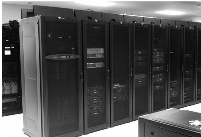
Fig. 3.12. Top , HVAC infrastructure at the Smithsonian Herndon Center. Photograph by Martin Kalfatovic, distributed under a CC BY-NC-SA 2.0 license; bottom , server racks inside the Smithsonian Herndon Center. Photograph by Martin Kalfatovic, distributed under a CC BY-NC-SA 2.0 license.
