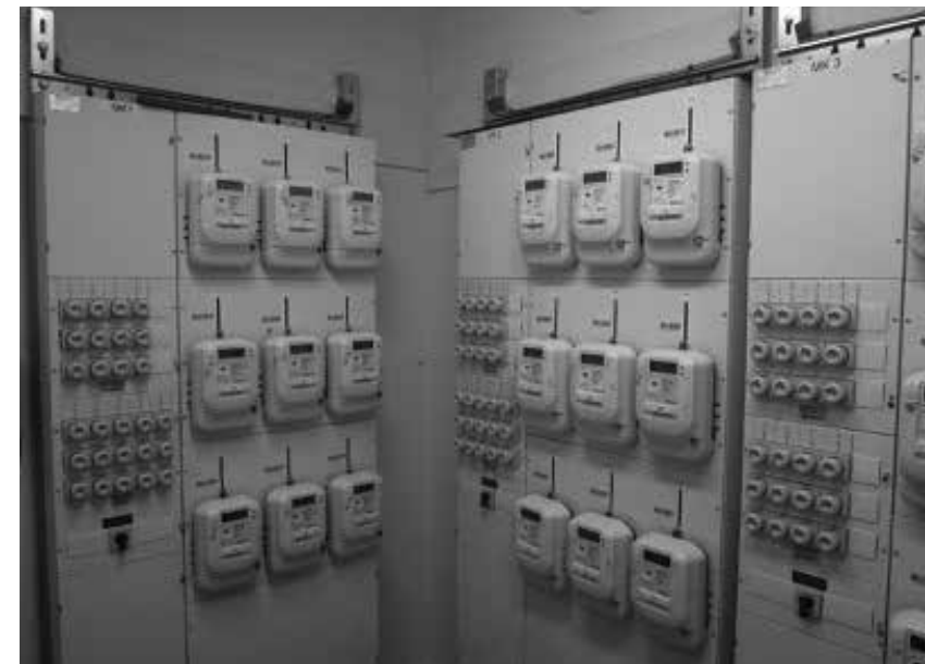
Fig. 4.8. Smart Meters locked up inside a central electricity room in the basement of an apartment building in Rihimäki, Finland.
