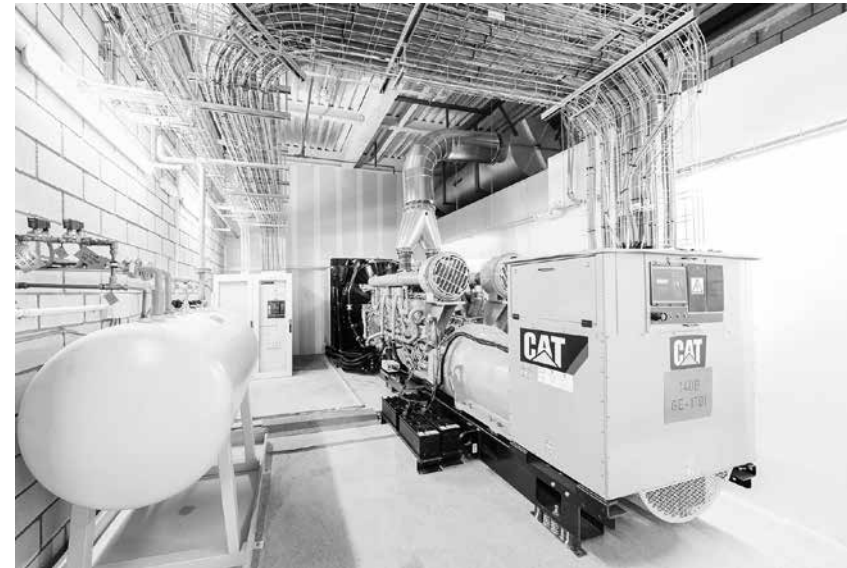
Fig. 1.11. Backup diesel generators inside a Data Center. Photography by Timo Arnall. All copyrights belong to Timo Arnall. Downloaded from http://www.elasticspace.com/2014/05/internet-machine in March 2016.
