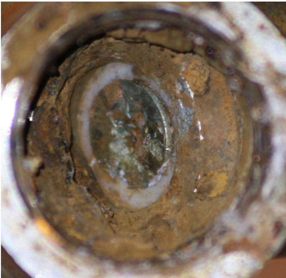
Figure 8. Corrosion and scaling in valve 9 reactor side.
