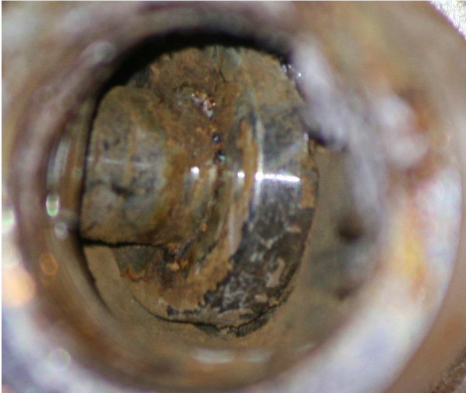
Figure 7. Corrosion and scaling in valve 9 CO 2 side.
