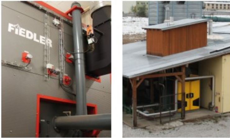
Figure 34 Furnace (left) and Triogen ORC (right) installed in Slovakia
