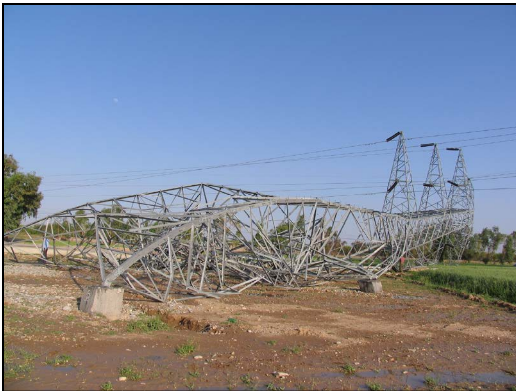
Figure 4.15 Under Service Tower Failure [19]
