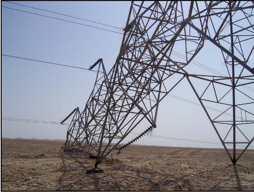
Figure 4.21 Tower Failure caused by unbalanced load [19]
