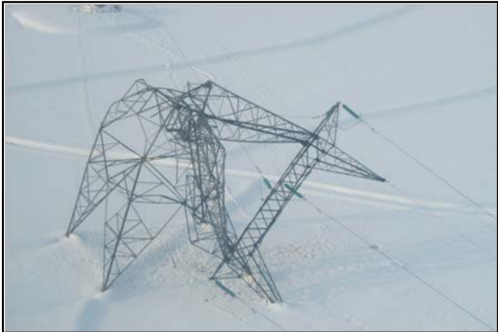
Figure 4.23 Tower Failure caused by harsh weather condition -2 [19]
