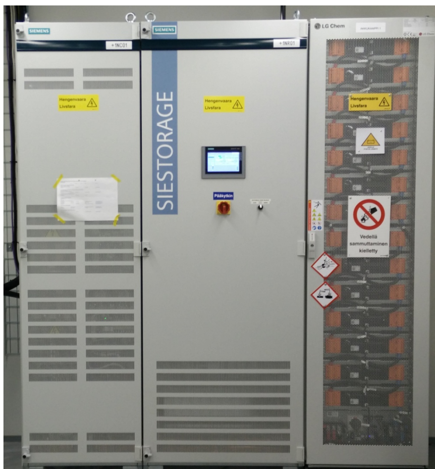
Figure 24: The Siemens SieStorage BESS in Viikki Environment House in Helsinki.
