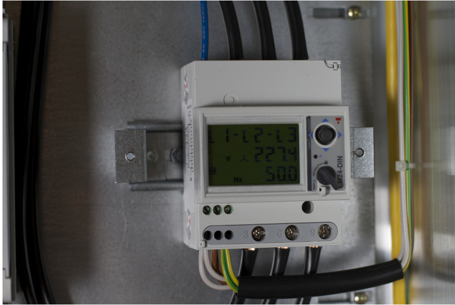
Figure 17: A Carlo Gavazzi EM24-DIN energy analyzer with the RS485 and some of the high voltage connections exposed.
