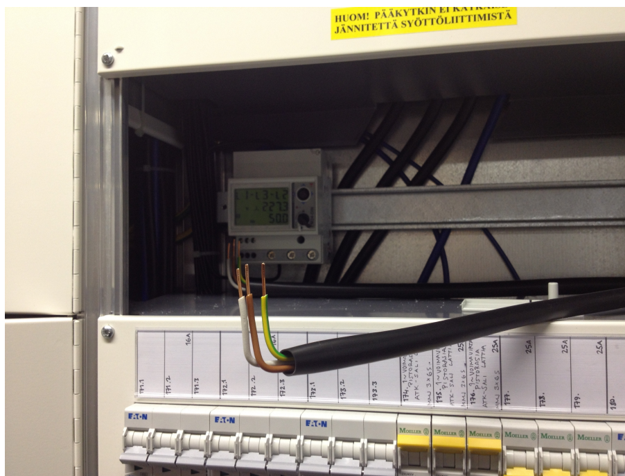
Figure 16: The two data wires and ground wire of an RS-485 bus, with another set of RS-485 wires and a Carlo Gavazzi EM24-DIN energy analyzer in the background.
