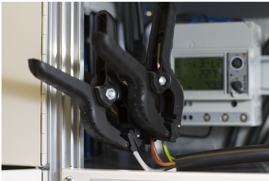
Figure 18: Bypassing a suspected faulty energy analyzer with photographers' clamps.
