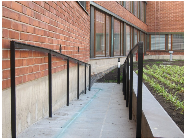
Figure 14. New accessible entrance to A wing with a push button switch. Aalto University/Antti Raika
