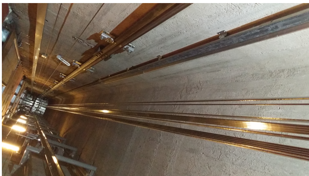
Figure 27: The concrete elevator shaft of Hyvinkää. Light ropes and the metallic ceiling of the shaft are seen in the figure.
