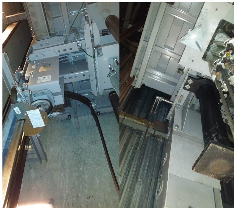
Figure 26: Bottom of the elevator car in Hyvinkää is presented on the left and the bottom of the car in Tytyri is on the right side of the figure. The radar corner reflector is attached to the bottom of the elevator car of Tytyri.
