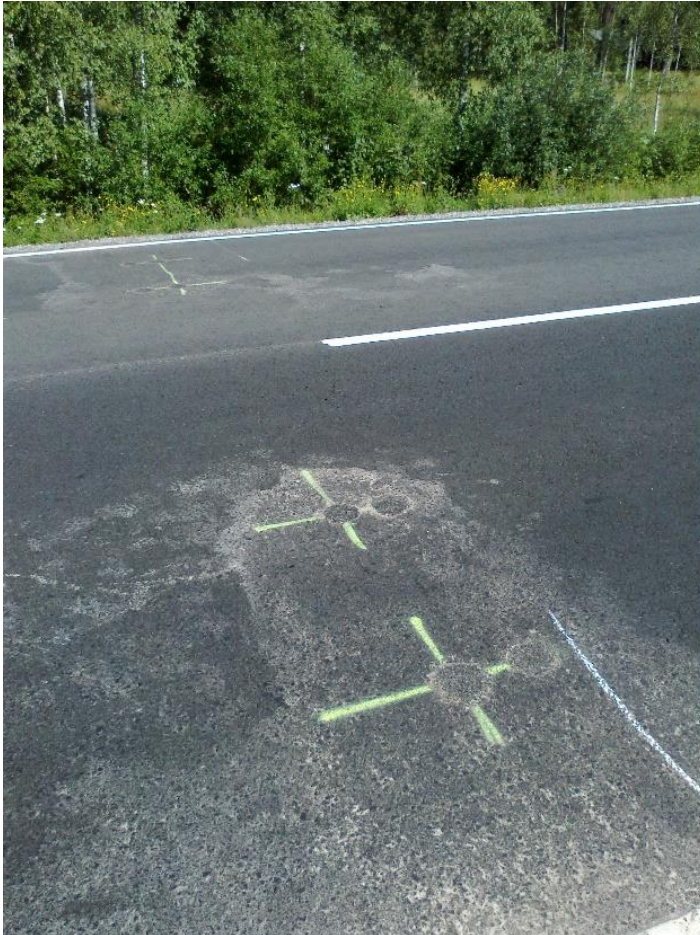
Figure 14: Asphalt samples were drilled from the right wheel path and between the wheel paths. The picture shows samples S2U_4420 and S2K_4420 in the front, and samples S1U_4420 and S1K_4420 on the other lane. Two samples were taken next to each other and named a and b
