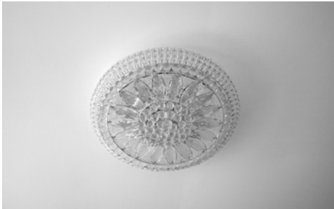
FIG. 05 The circular flush mount type lighting fixture in the living room of the Souzas.
