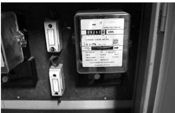
FIG. 15 The ‘Delivery of Measures’ was carried out through manual recording of energy consumption measures from domestic electricity meters in the basement of the apartment block.
