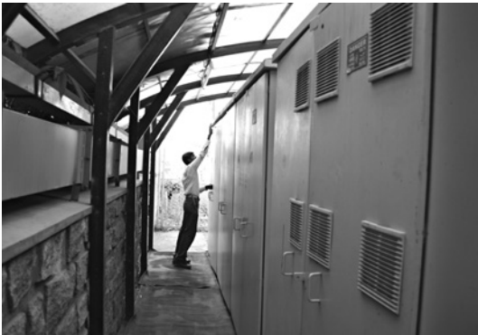
FIG. 04 Madan opening the door of a meter housing in the electric yard.
