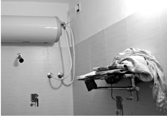
FIG. 10 The hot water electric geyser in Dr Shenoy's bathroom.
