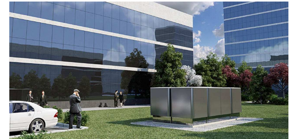
Figure 33. Bloom energy Server installed into courtyard.
