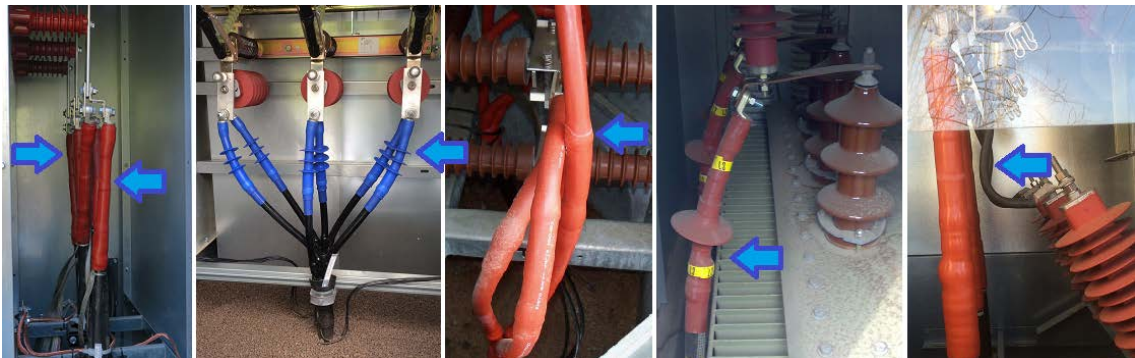
Figure 23: Problematic installations from real life
