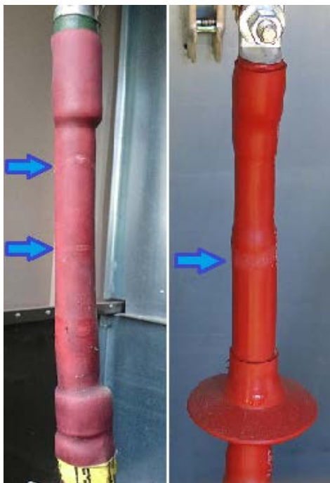
Figure 14: Faint marks of dry band arcing on termination surfaces
