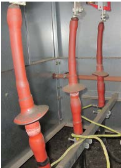
Figure 21: Severely polluted terminations inside a secondary outdoor substation
