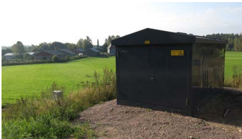
Figure 19: Conventional secondary outdoor substation located in the countryside
