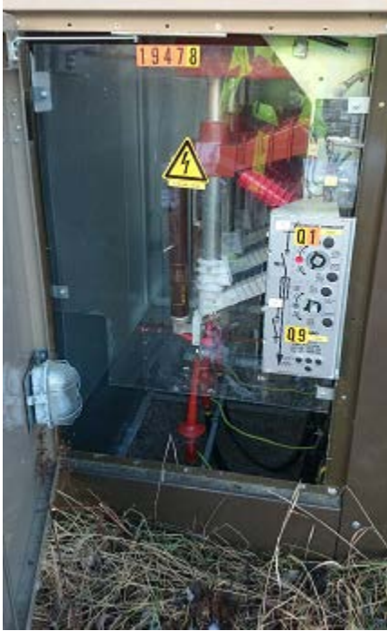
Figure 22: Partially submerged structure with terminations below ground level
