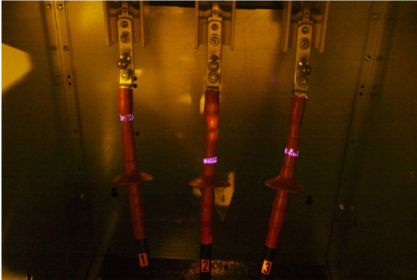
Figure 15: Visible dry band arcing in 20 kV indoor terminations
