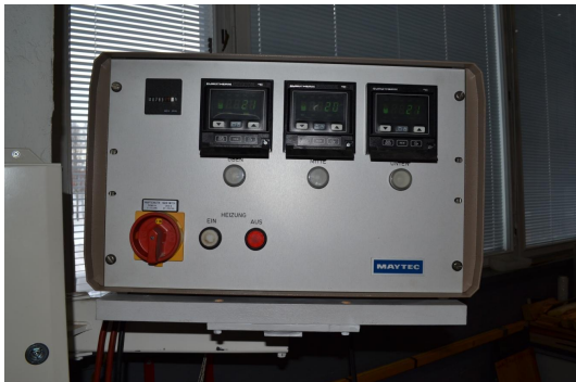
Figure 3.7 Controlling unit of furnace
