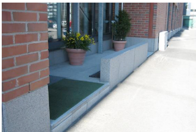
Fig 12 Step is too high.
