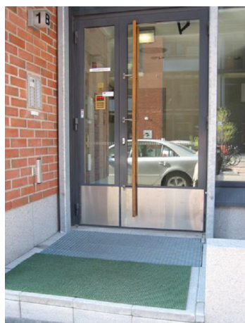
Fig 11 Door opens in wrong direction.
