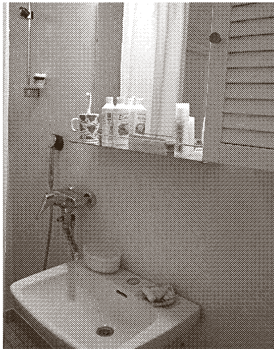
FIGURE 6.2 Pictures from an original 1950s bathroom to be renovated in As Oy Planning (photos by a dweller at As Oy Planning, P65, 2, 6, 7). Residents wonder about the different options for renovation and costs for them.
