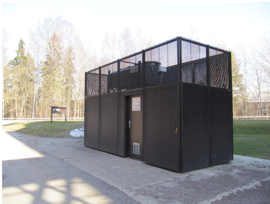
Figure 8: A photo of the cooling unit that utilizes rooftop fans to cool the liquid that is used in the data center by the CRAC and water cooled cabinets.
