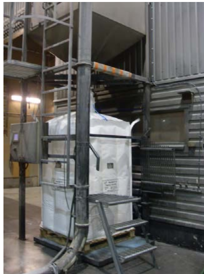
Figure 17. Plastic granulates are poured from the silo into sacks. One sack contains 1000 kg recycled plastics.
