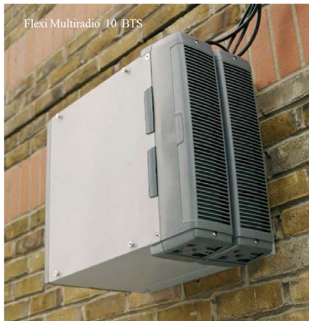
Figure 1. Nokia Flexi Multiradio 10 Base Station mounted on wall. Base stations are mainly produced from aluminium but they also contain plastics. (Nokia Networks 2014a)
