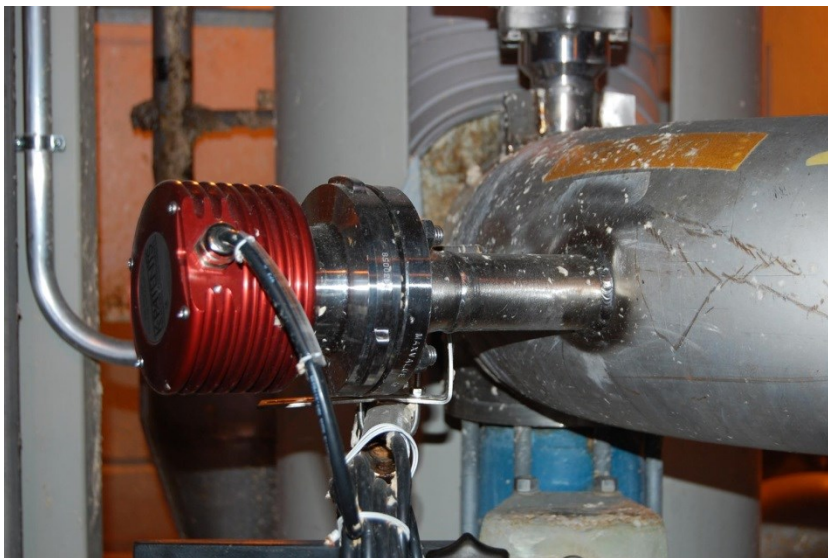
Figure 23. Installation of the PR-23 refractometer in feed pulp line of DD3.
